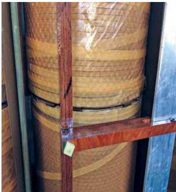
Photo 1 - Insufficient Cooling of Windings Resulting in Thermal Failure
