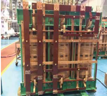
Photo 16 – Good Practice of LV Bus Bars Anchoring.
