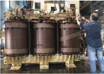
Photo 10 - Inadequte Mechanical Supports for Short Circuit Forces
