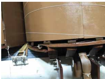
Photo 7 - Inadequate (Improper) Mechanical Support
