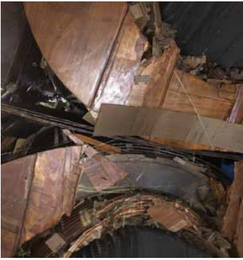
Photo 8 - Poor Quality of PW Rings
