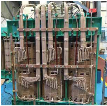
Photo 15 – Good Practice Of Lead Routing And Coils Anchoring
