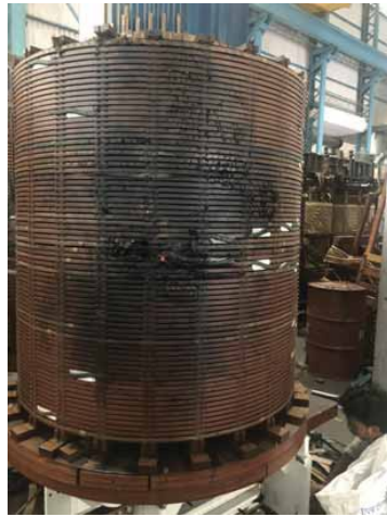
Photo 11 - Dielectric Failure Resulting in Short Circuit Failure In HV Windings
