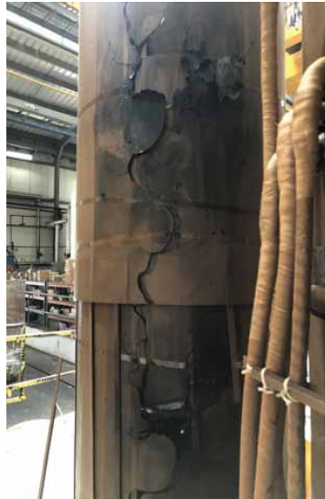
Photo 14 - Dielectric Failure of Insulation System due to over Voltages
