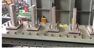
Photo 16 – Fibre Glass Bushings for LV (High Current).
