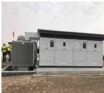
Photo 5 - Impair of natural cooling due to blockage from inverters mounted close to the transformer
