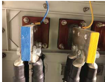
Photo 3 - Breaking And Leakage From LV Epoxy Bushings
