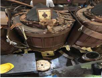
Photo 9 – Failure of LV Windings in all three Phases under Dynamic Inabiltiy to withstand Short Circuit Forces
