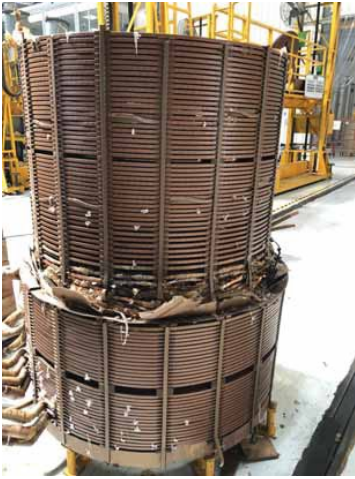
Photo 12 - Dielectric Failure Resulting in Short Circuit Failure of Windings
