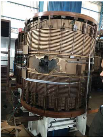
Photo 13 - Dielectric Failure of HV Windings due to over Voltages
