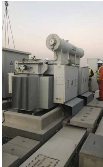
Photo 2 - Insufficient Cooling of Total Losses Generated
