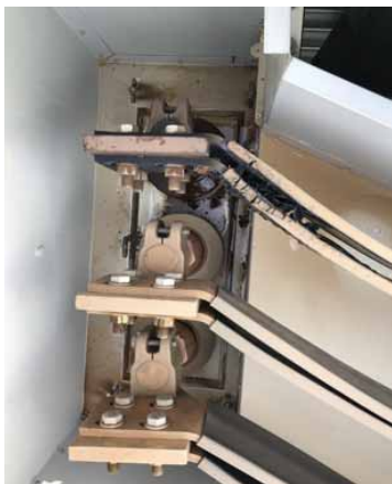
Photo 6 - Burning Of Lv Side Bus Bar Sleeve Due To Insufficient Cooling (Bus Duct Blocking The Heat Dissipation)
