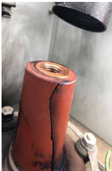
Photo 4 - Failure of HV Elastimould Bushing due to Inadequate Creepage Distance
